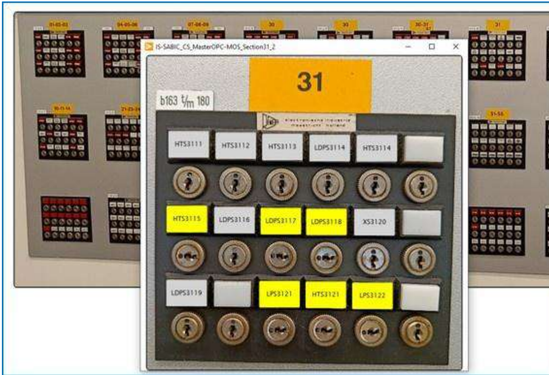
Replica of Key Override in Control Room
