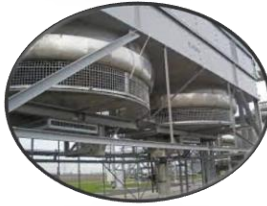
Air-Cooler Heat Exchanger 12
