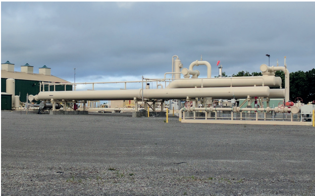
Size slugcatcher and define its control strategy based on rigorous multiphase simulation
