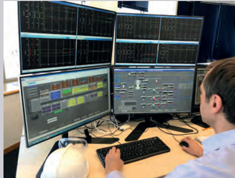
HMI checking before commissioning
